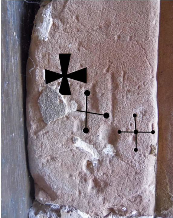
Fig 2: Combined cross pommée and cross pattée marks on the south-east door jamb at St Mary's, Shrawley (author's photo)
